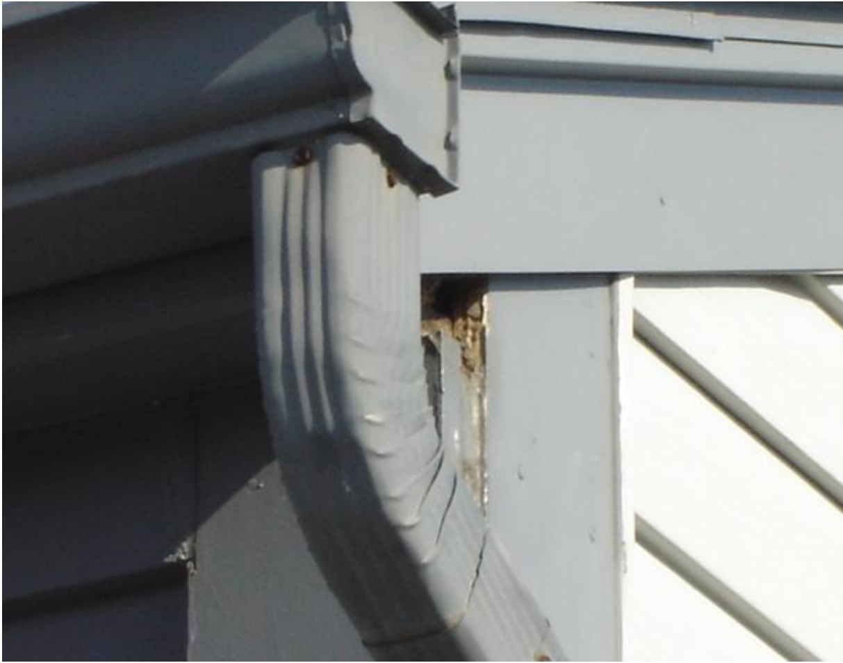
Sparrow(s) were entering/exiting at SE upper corner fascia area/opening.
