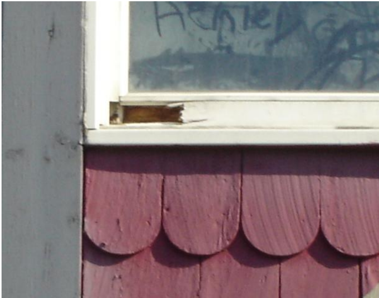
Window & frames in need of repair or replacement as necessary.
