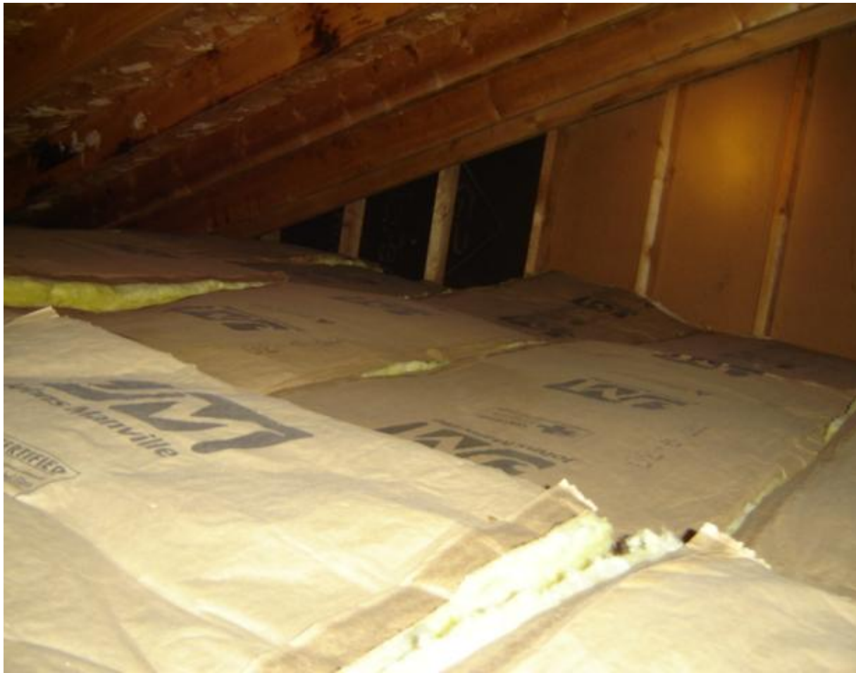
Batts Insulation: Vapor barrier/kraft paper is installed improperly with the vapor barrier on the top side - it should be on the ceiling side or removed.
