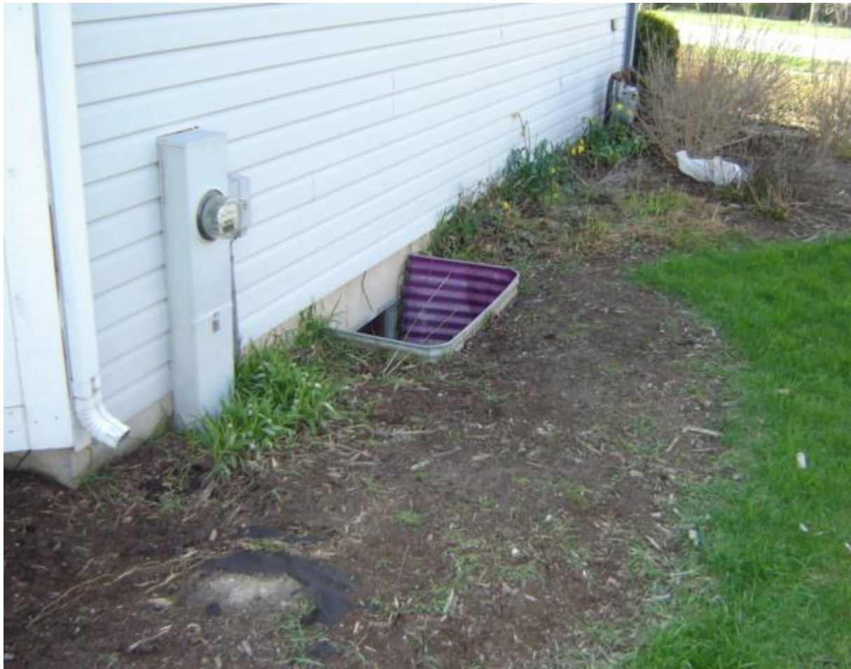
Low areas next to the foundation need some correction. Recommend additional backfill to create a proper pitch away from the house.
