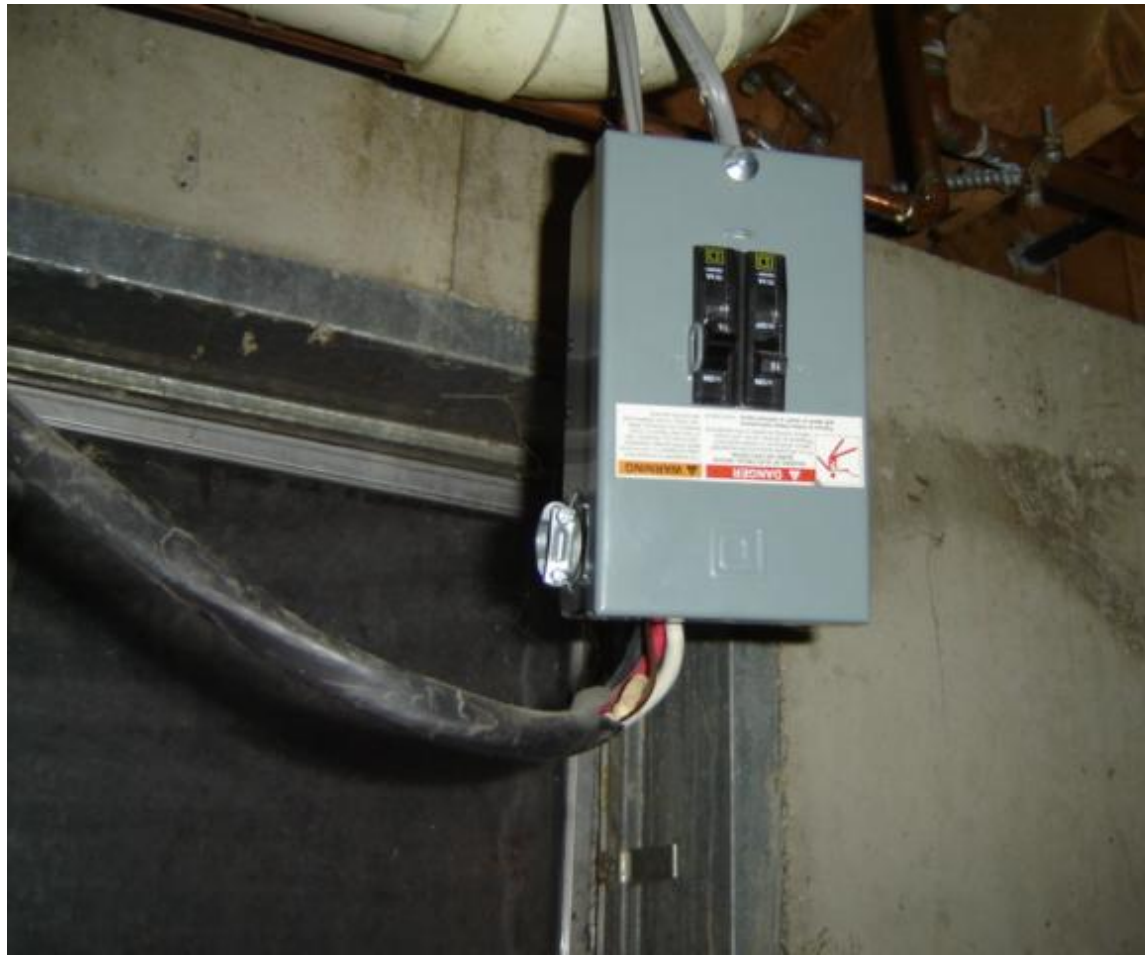
Sub-panel/box in laundry area needs to be properly secured (hanging).
