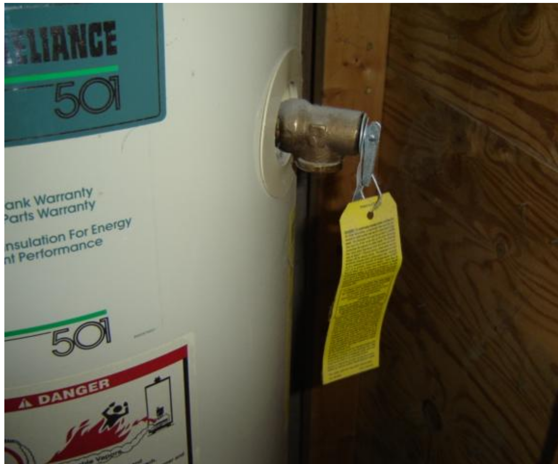
Temperature-Pressure relief valve extension is missing and needs to be 4"-6" off of the floor - this is a Safety Concern.
