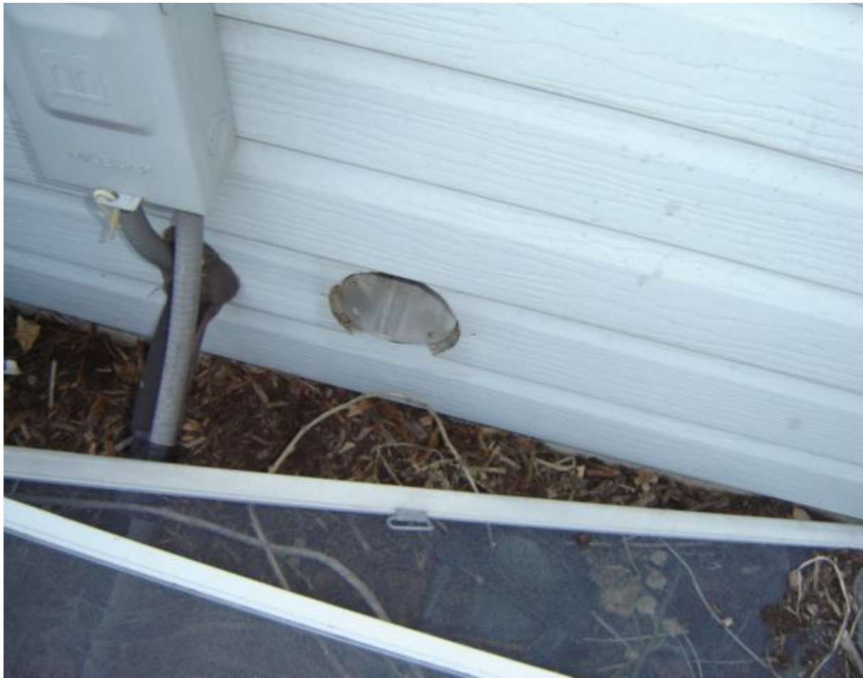
Exterior dryer vent is missing cover.
