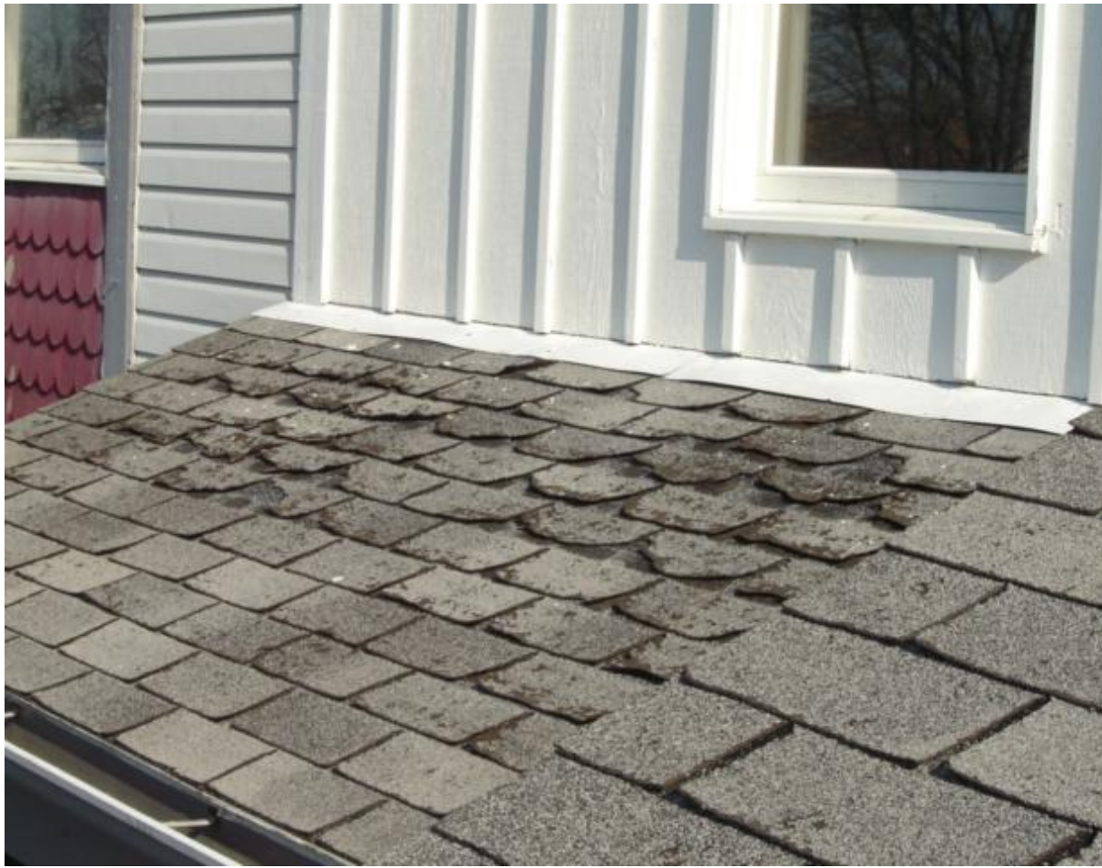
Roof was in poor condition and will need repair and/or replacement soon.
