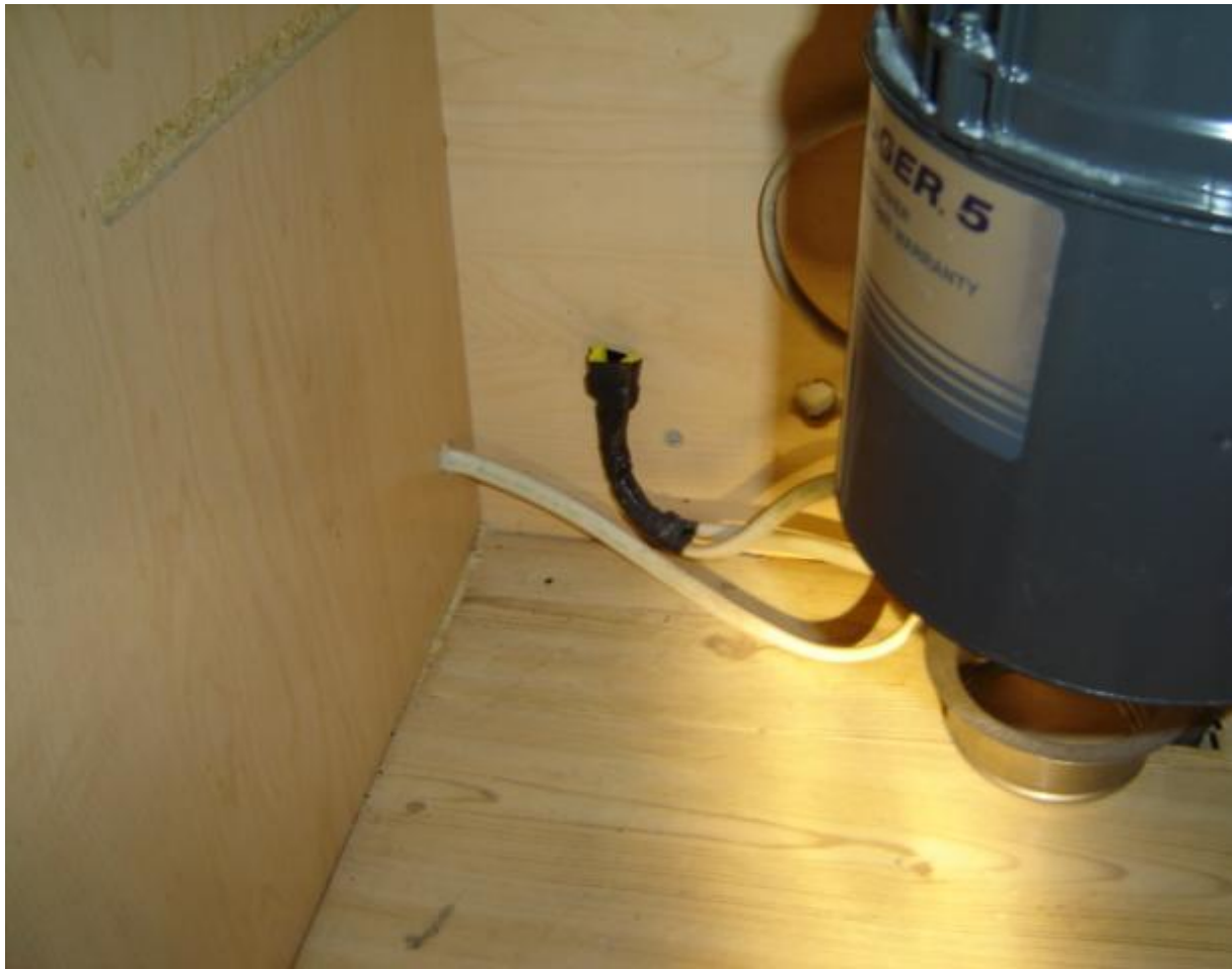
Spliced romex present under kitchen sink; recommend a junction box.
