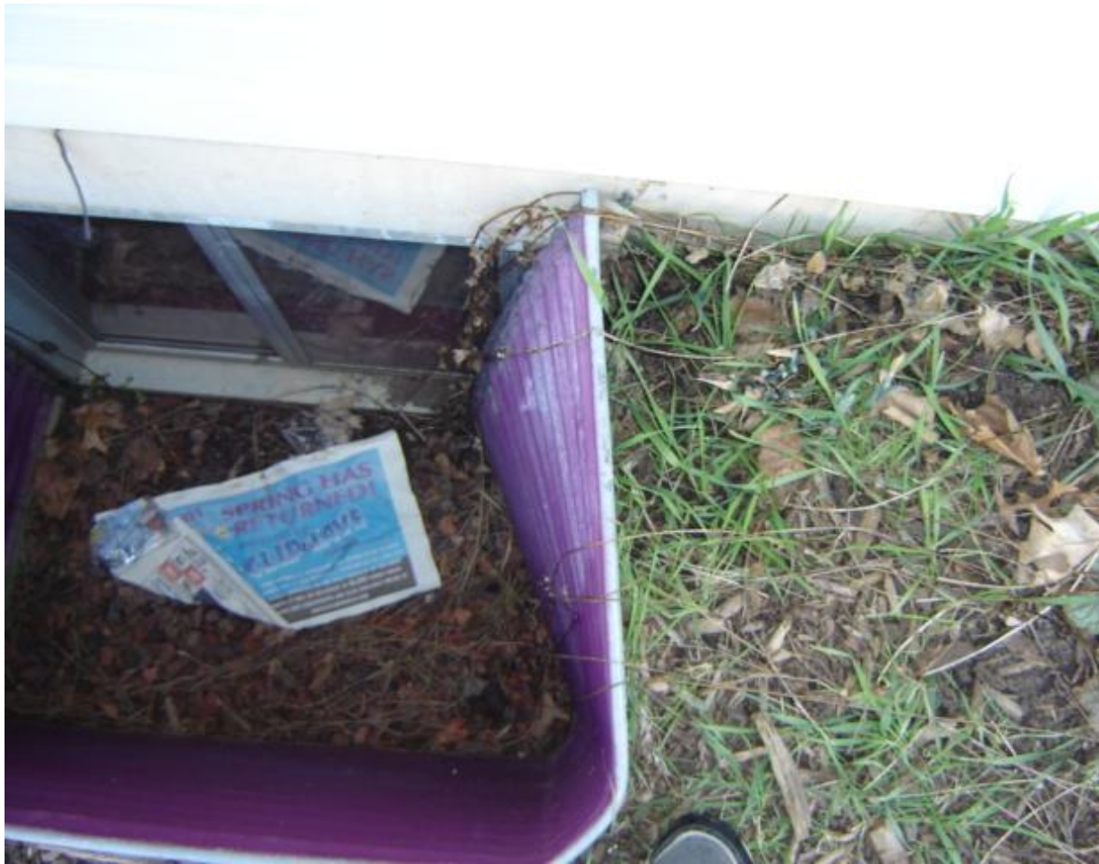
West window well needs to be reset; currently bowing inwards.
