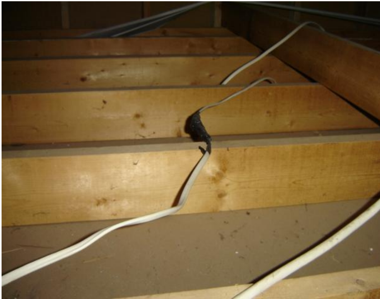
Spliced romex present in garage attic; recommend placement in a junction box.
