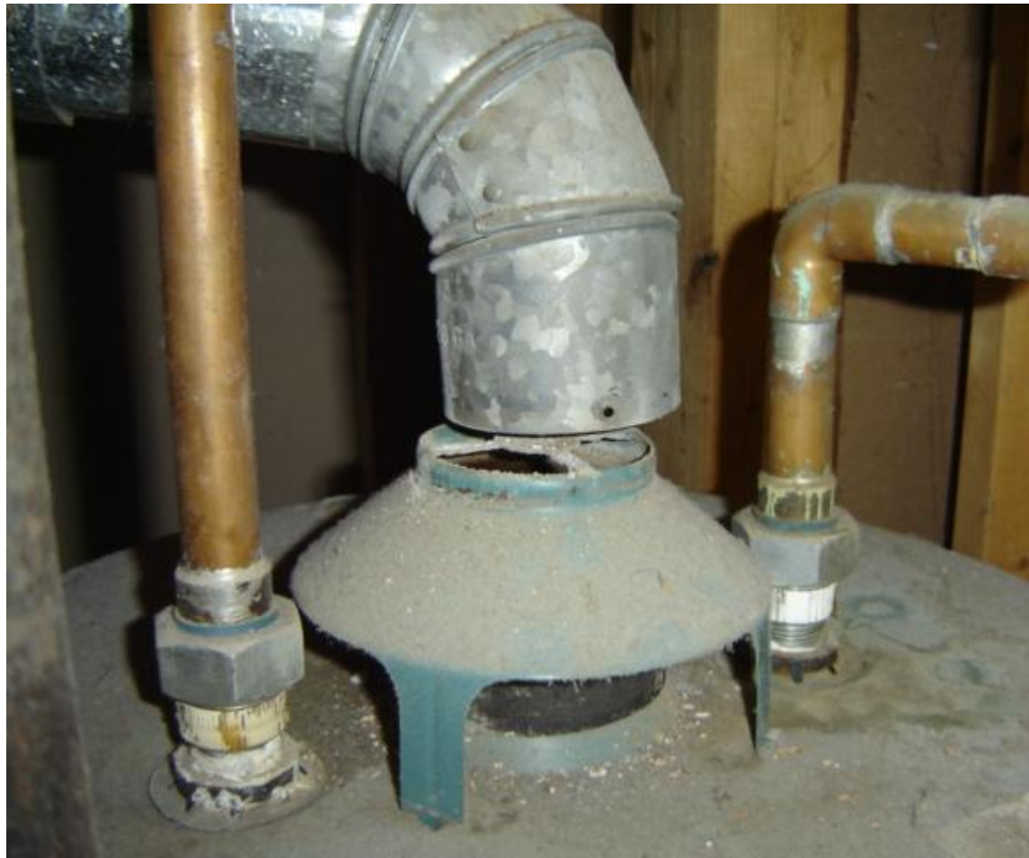
Water heater flue/draft hood need to be properly secured (screws added).
