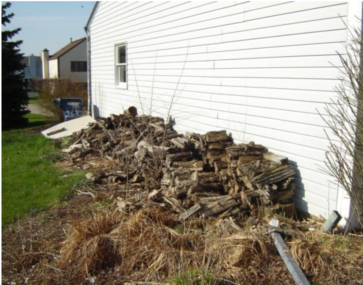
Recommend moving/relocating wood pile away from house.
