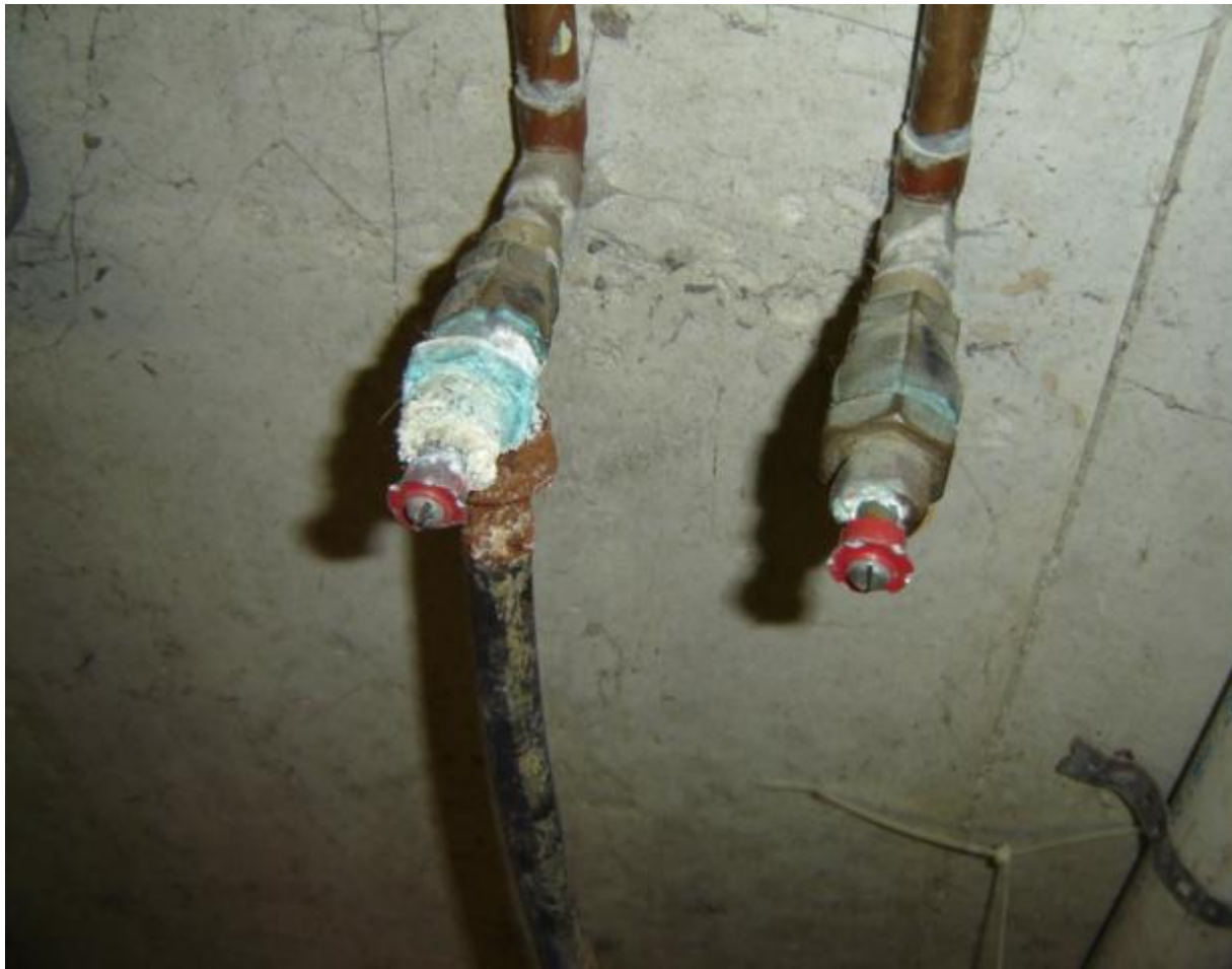
Laundry shut off valves are broken.
