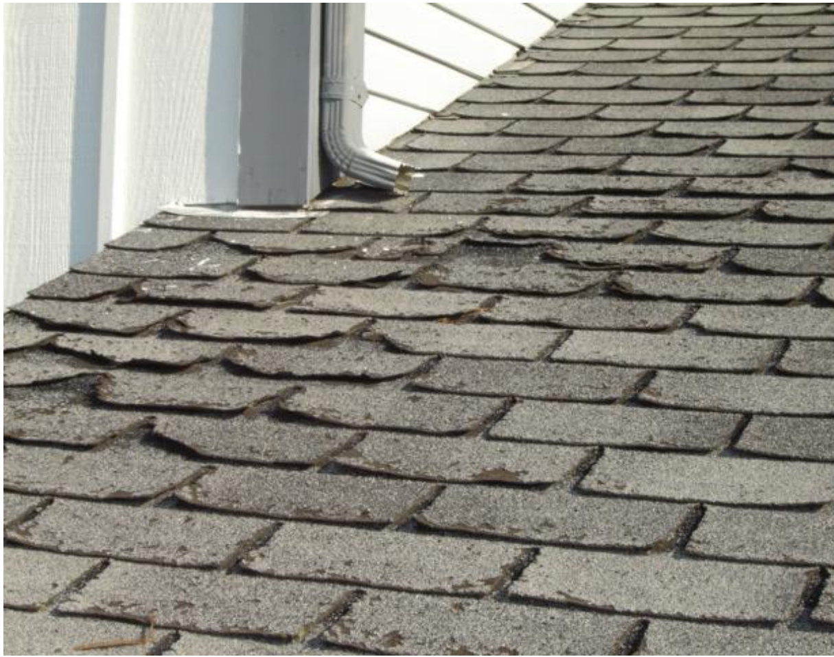
Roof was in poor condition and will need repair and/or replacement soon.
